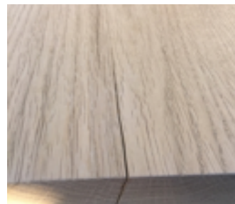
On table tops with wide and thick sticks, small cracks may appear, especially at the end of the table top. It often occurs in the winter months, where it is cold and the air is dry. Most often, these will retract again during the summer months. Because of the extremely wide planks on the TREE TABLE, cracks are inevitable and they might not retract again.
